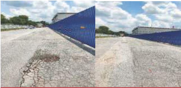
4. Difficult road condition (Road damage and potholes lane road)
